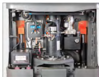
MOSFET control system
